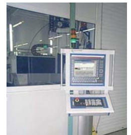
Machine control panel
