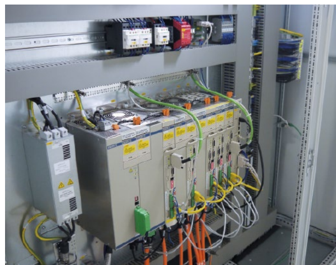
Detailed view of control cabinet: Flexium+ 68 CNC system with NUMDrive X with integrated safety solution.
