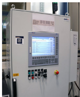
Optimized HMI after retrofit
