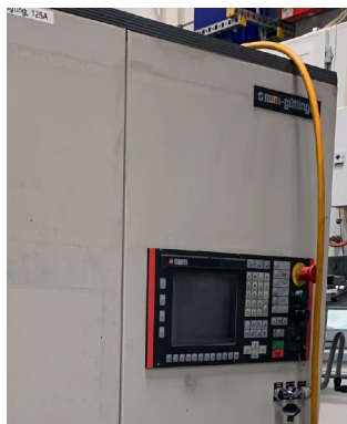
HMI before retrofit
