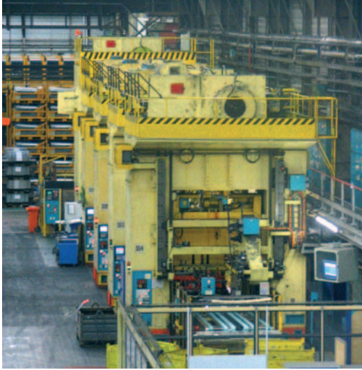
The 300 stamping line includes five presses, one 475 ton press and four 400 ton presses, a blank destacker and four inter-press islands, the whole comprising 28 axes and nearly 1800 inputs/outputs.
