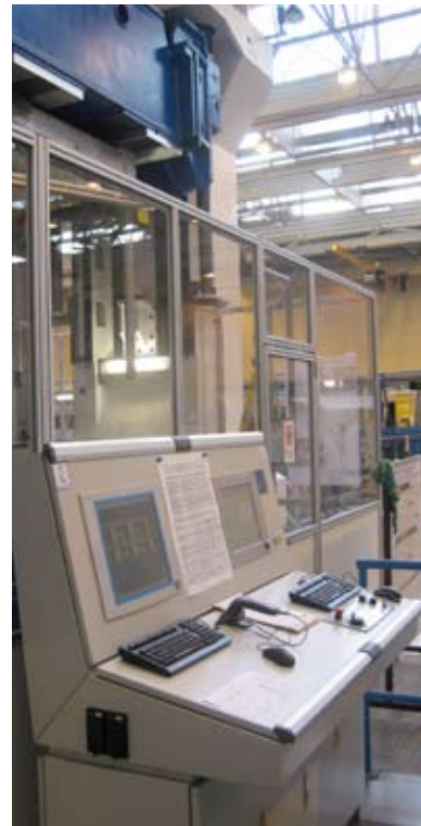
The control desk
