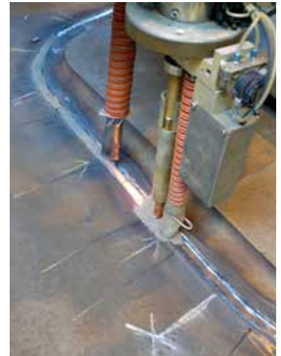
Top: SA system during welding process – the system moves to the pre-defined teach points
